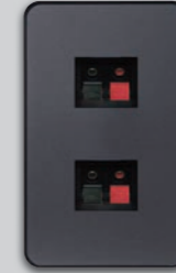
스피커 잭 2구 Speaker Jack C-WIRING-2C1D CPRTP11021DP (대각 PLATE 2구)
